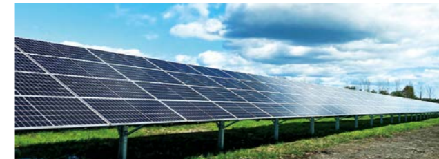
Solar panels placed on Kushiro Factory
