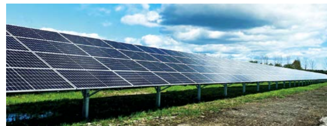
Solar panels placed on Kushiro Factory
