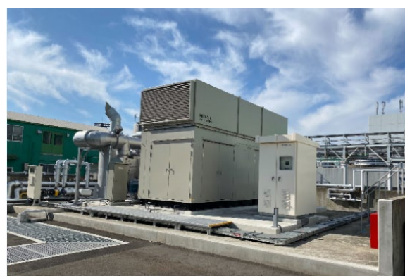
Naruto Factory's cogeneration system
