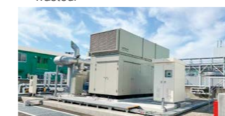
Naruto Factory's cogeneration system
